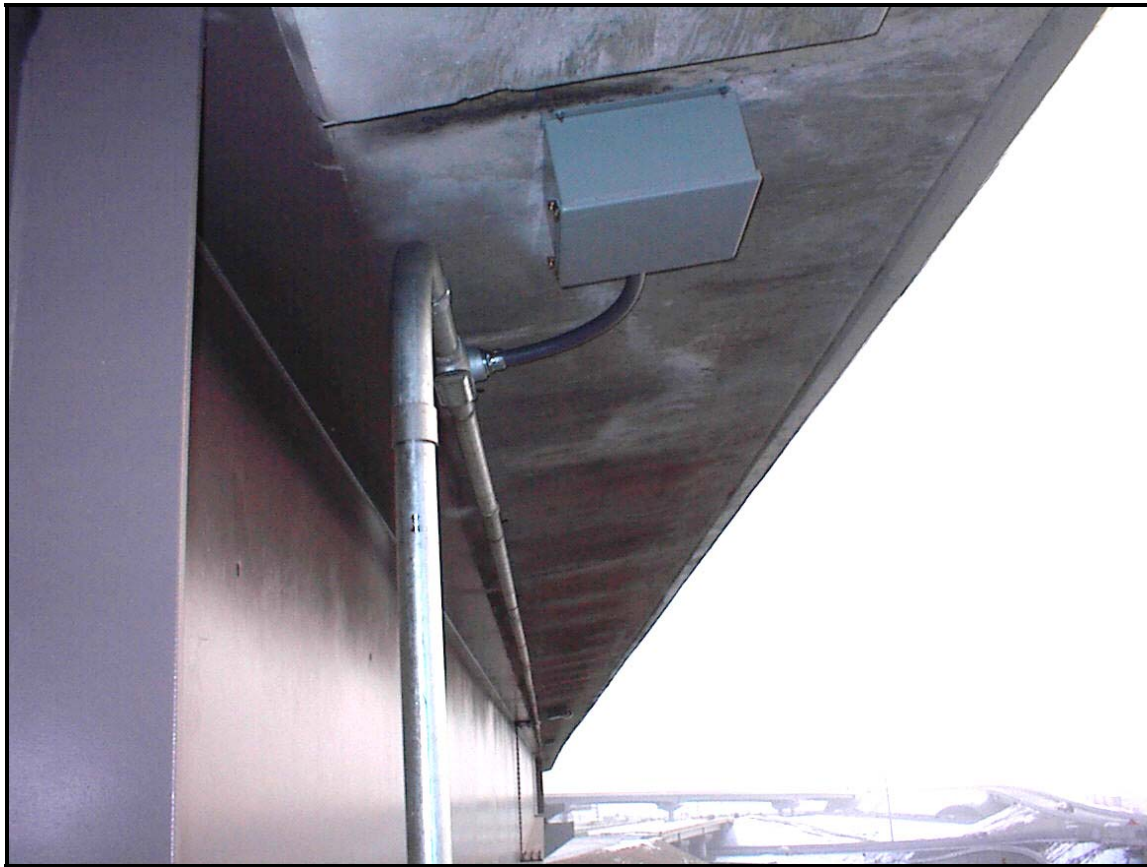
FIGURE 8 Box mounted on bottom of deck
