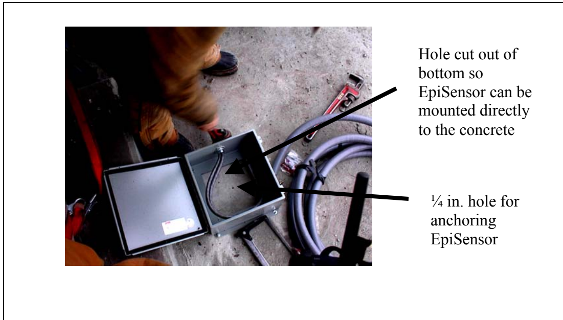
FIGURE 10 Nema 12 enclosure installation
